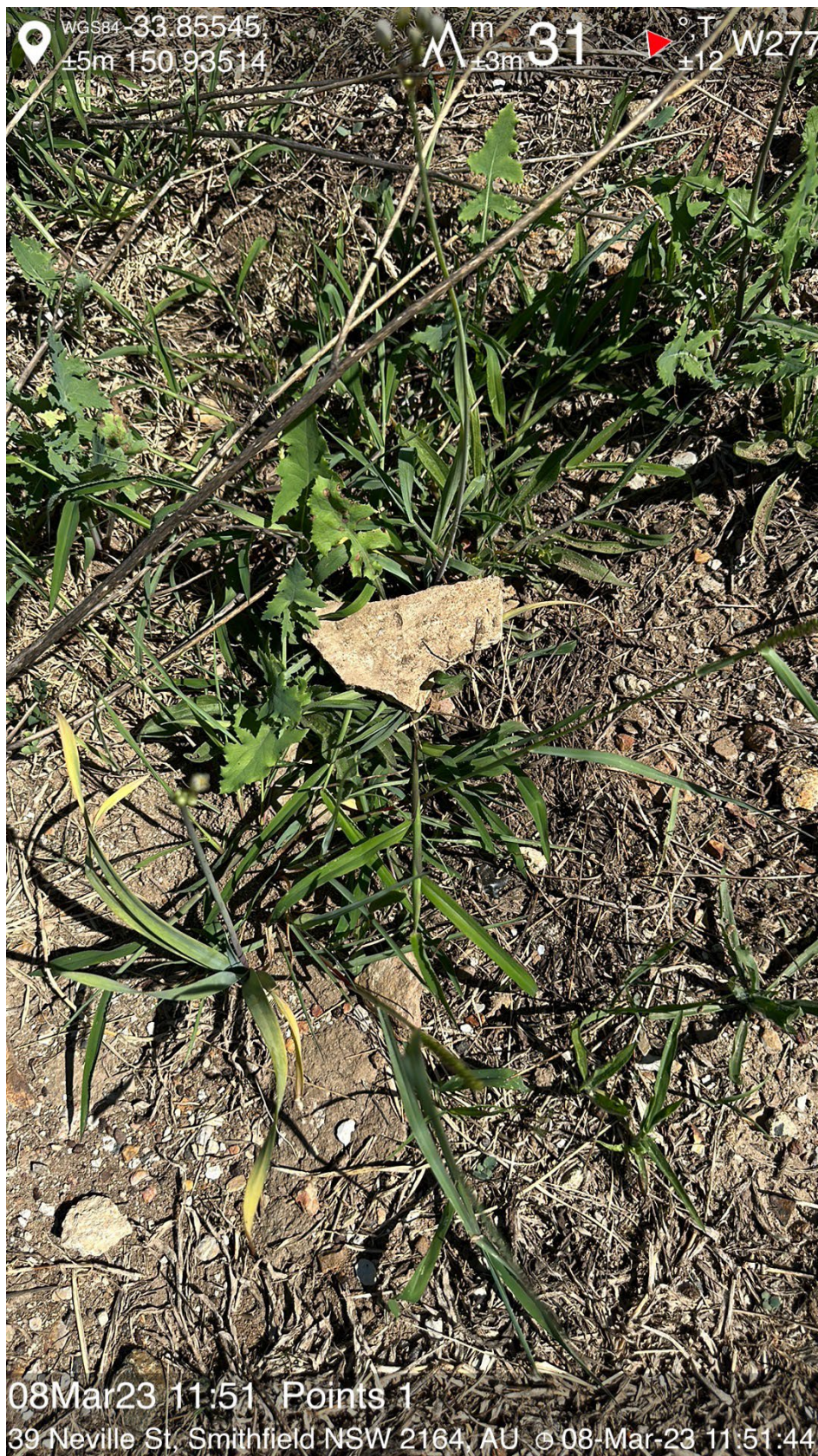
Plate 23: Example of potential ACM observed on the surface in this part of the site.
