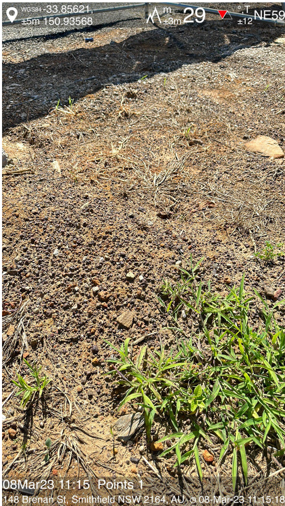
Plate 46: Example of potential ACM observed on the surface in this part of the site.
