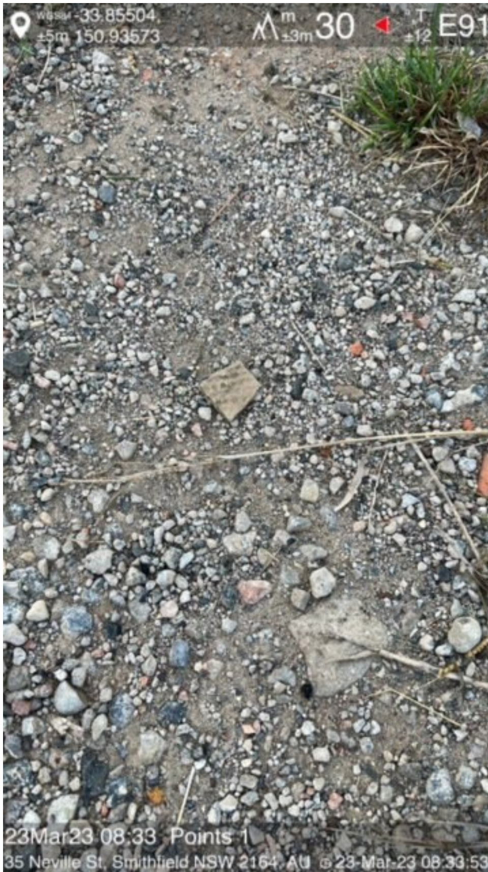
Plate 13: Example of potential ACM observed on the surface in this part of the site.
