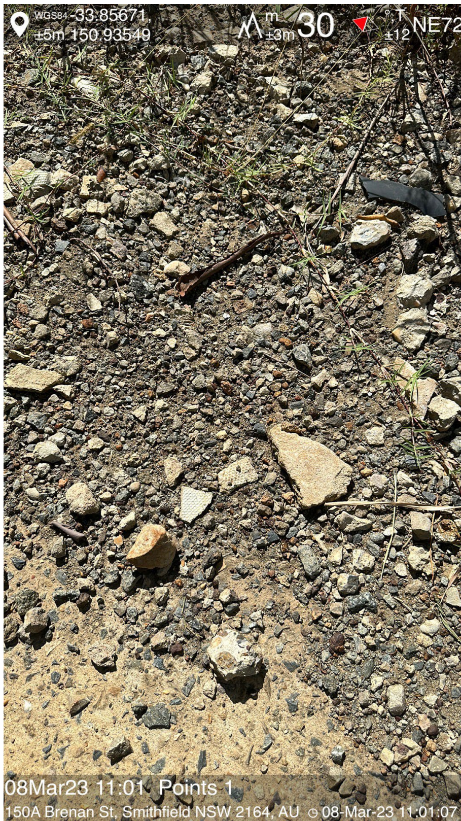
Plate 49: Example of potential ACM observed on the surface of 150a Brenan Street.
